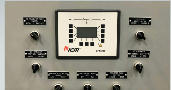
Transfer Switch XFER-200 controller and LCD display
